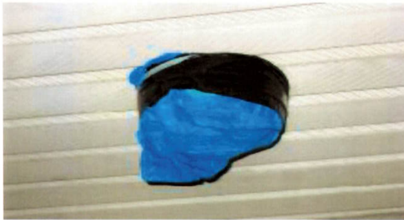
5.10.1 Figure 6: Bagged & taped smoke detector
